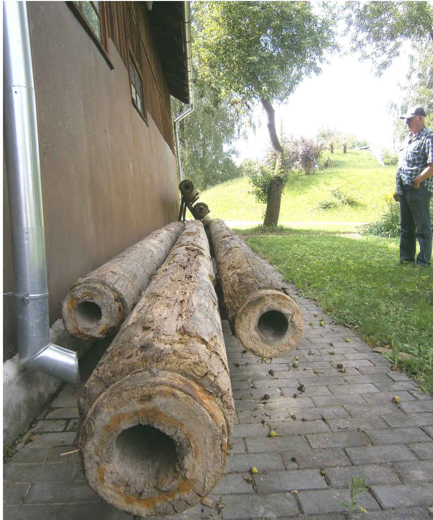
Figure 1. The water pipes of water-supply system in Jelgava
